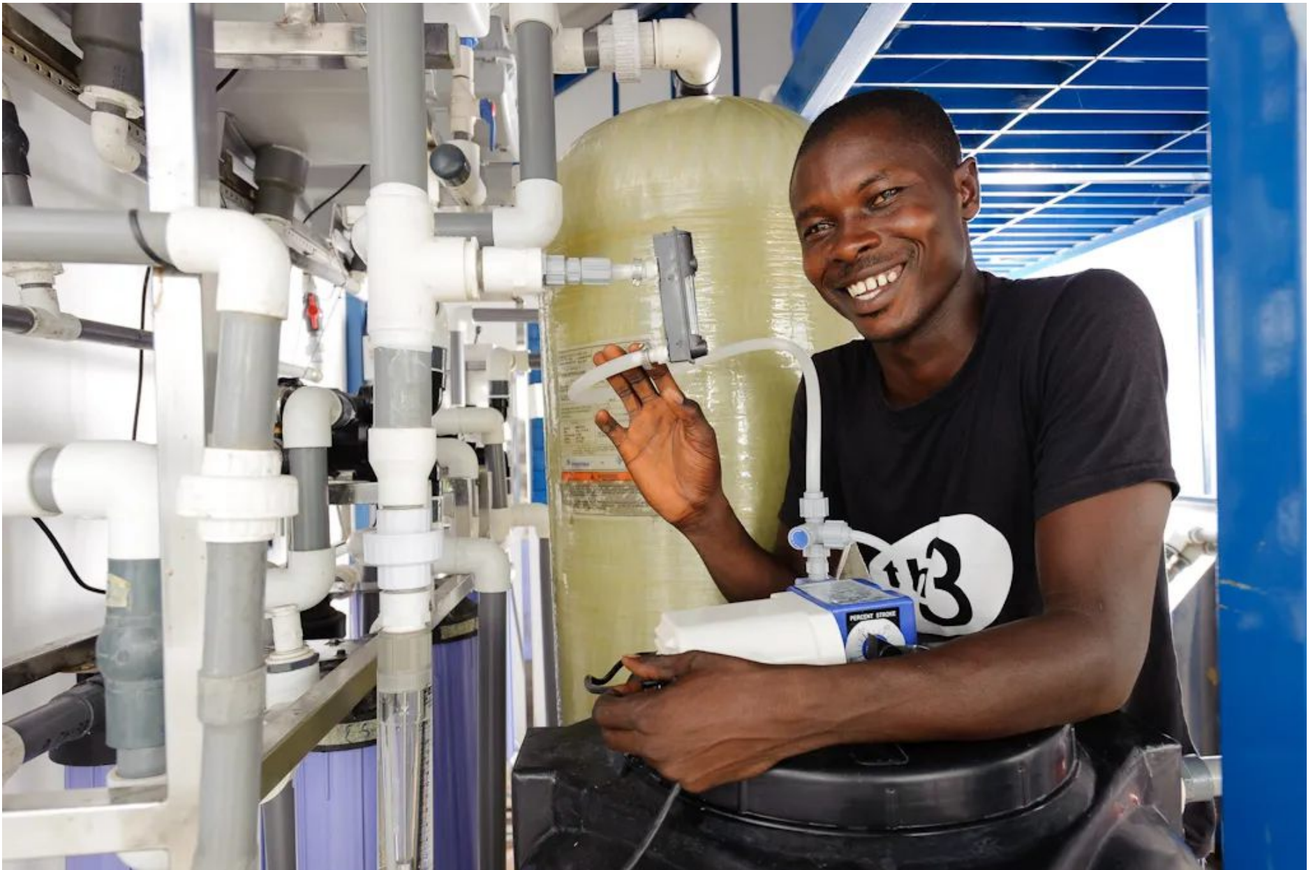
A WaterHealth Center operator monitors water quality in Adeiso, Ghana. Photo credit: The Coca-Cola Company
